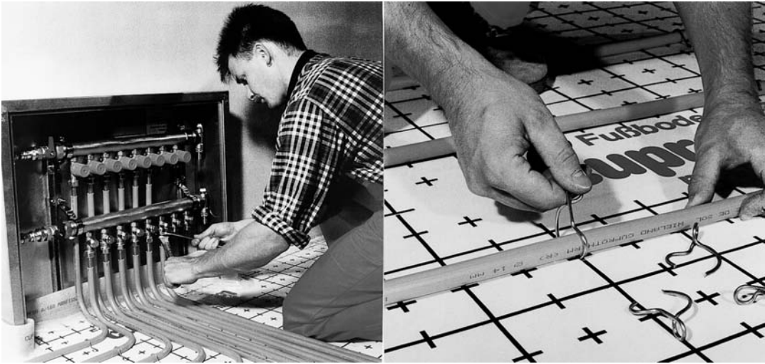
Fig. 2.85 Domestic insulation and under-floor heating in extruded and drawn (plastic-insulated) copper tubes. Source: Wieland-Werke AG
