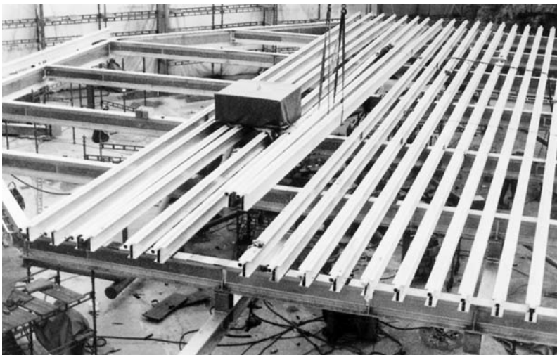
Fig. 2.75 Assembly of the supporting profiles shown in Fig. 2.74 for the helicopter landing platform. Source: Alusuisse
