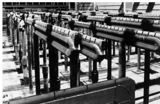
Fig. 2.90 Special sections as support tubes in a walking beam furnace for heating steel slabs
