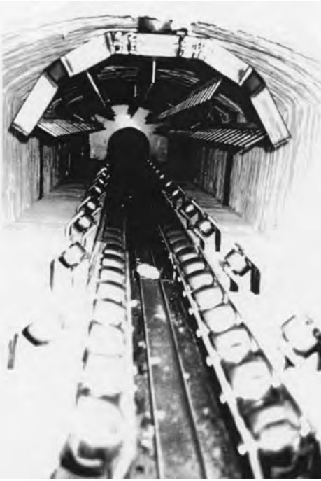
Fig. 6.47 Furnace tunnel of a rapid-heating gas-fired furnace with nozzle boxes and nozzles for preheating the billets by exhaust gas circulation
