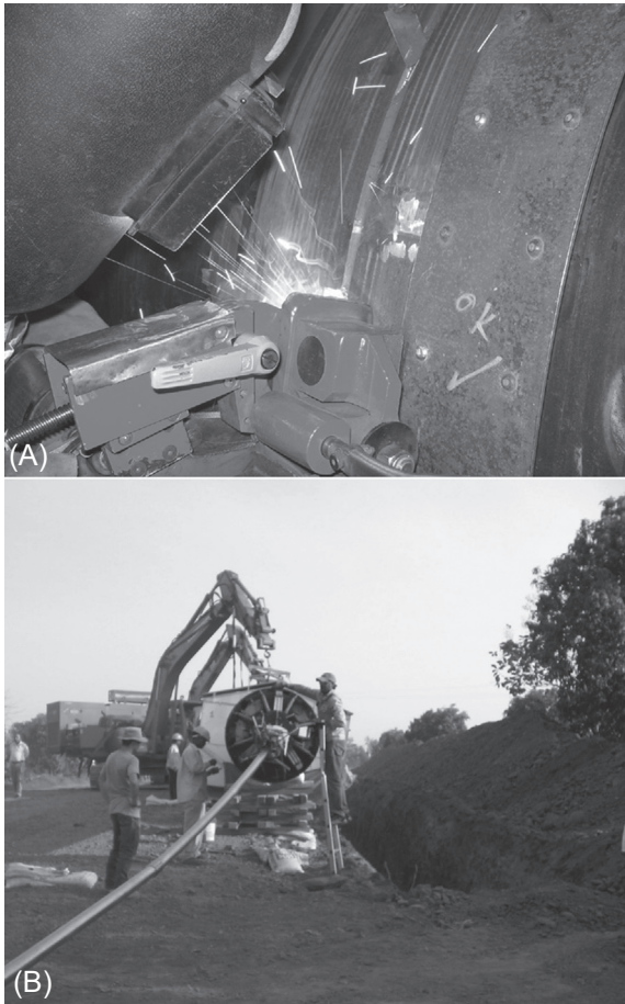
Figure 2-3-4 (A) Mechanized welding being performed; (B) mechanized welding of 48-in. diameter pipe.
